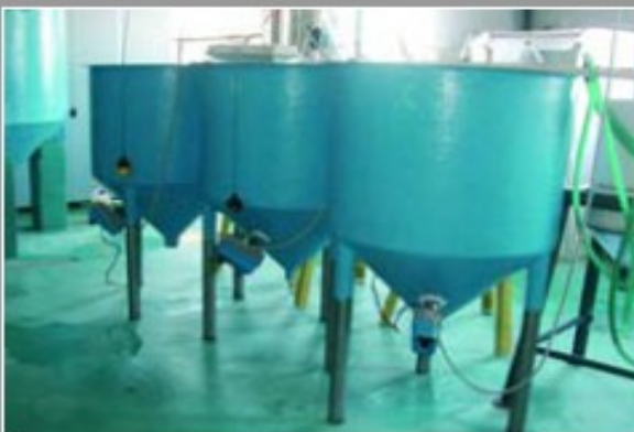
Fig. 83 - Tanks equipped with titanium heaters and thermostats
