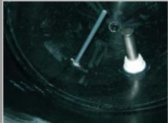
Fig. 84 - Internal view of tanks in Fig. 83: the heater and the thermostat probe
